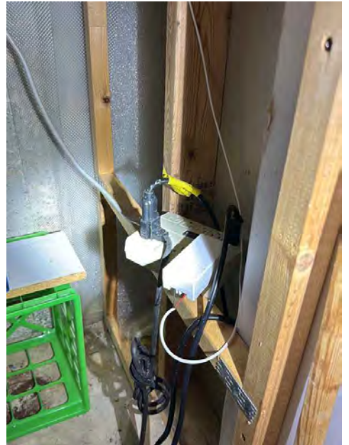
Surge protector not proper, suggest designated outlet
