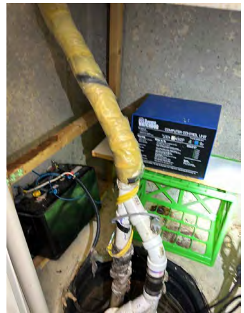
Battery not functioning, replacement needed
