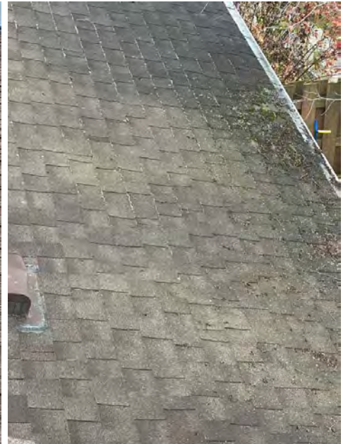
Have further evaluated and repaired
