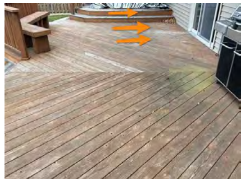
Have further evaluated and repaired if necessary
