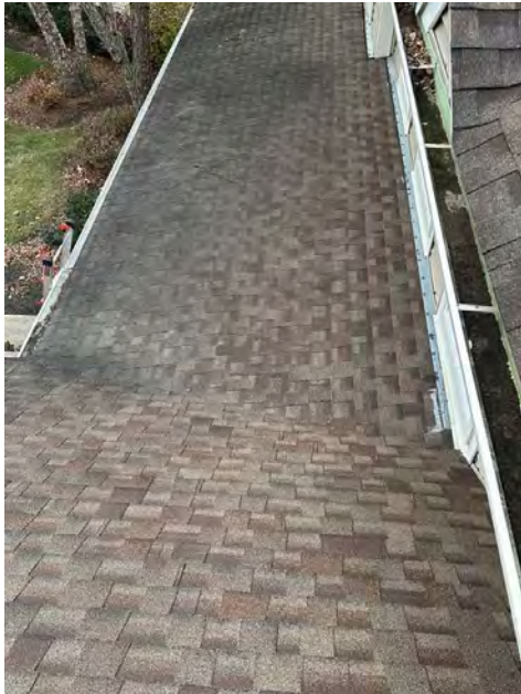
Have further evaluated and repaired
