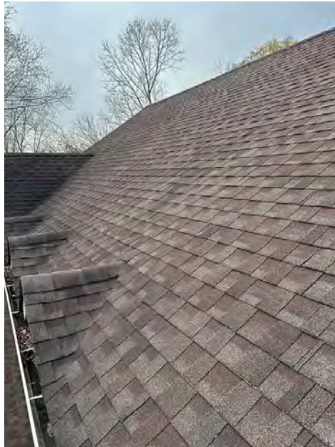
Have further evaluated and repaired
