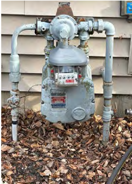
Main Fuel Shut-off
