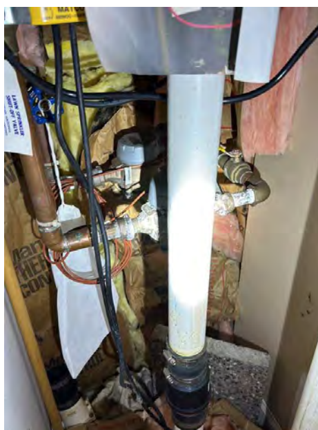
Main Water Shut-off
